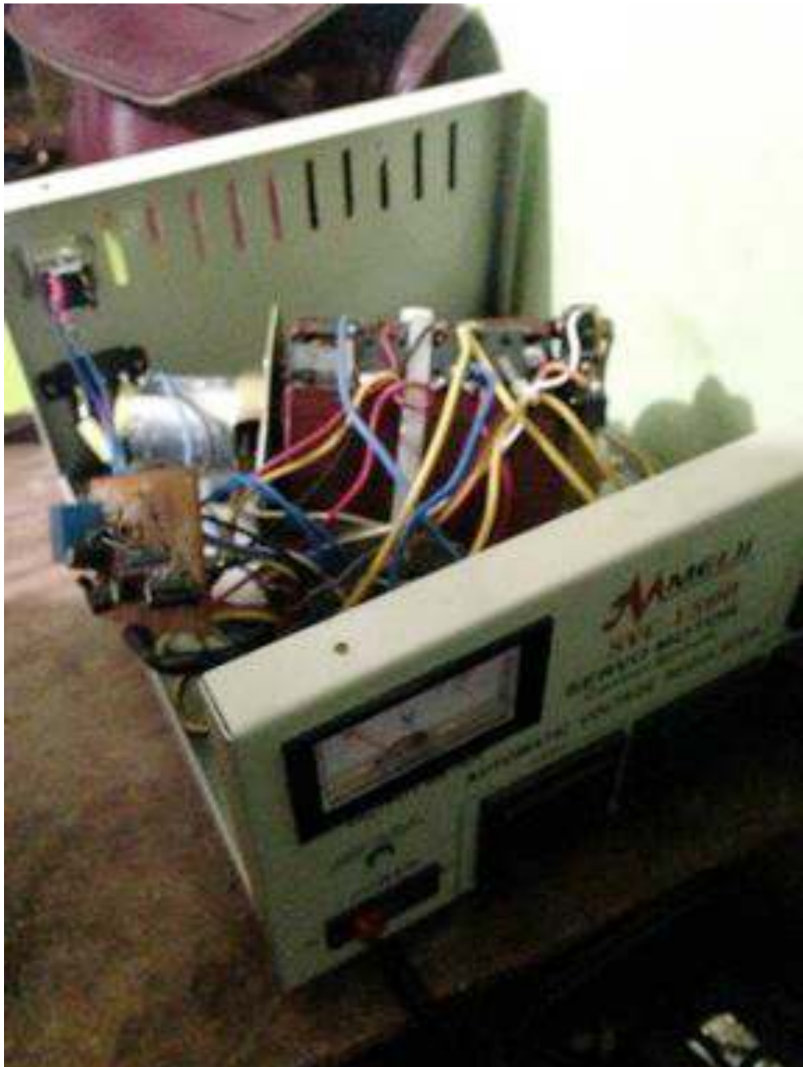
Figure 12: a broken Automatic Volume Regulator at the Radyo Bakdaw studio
